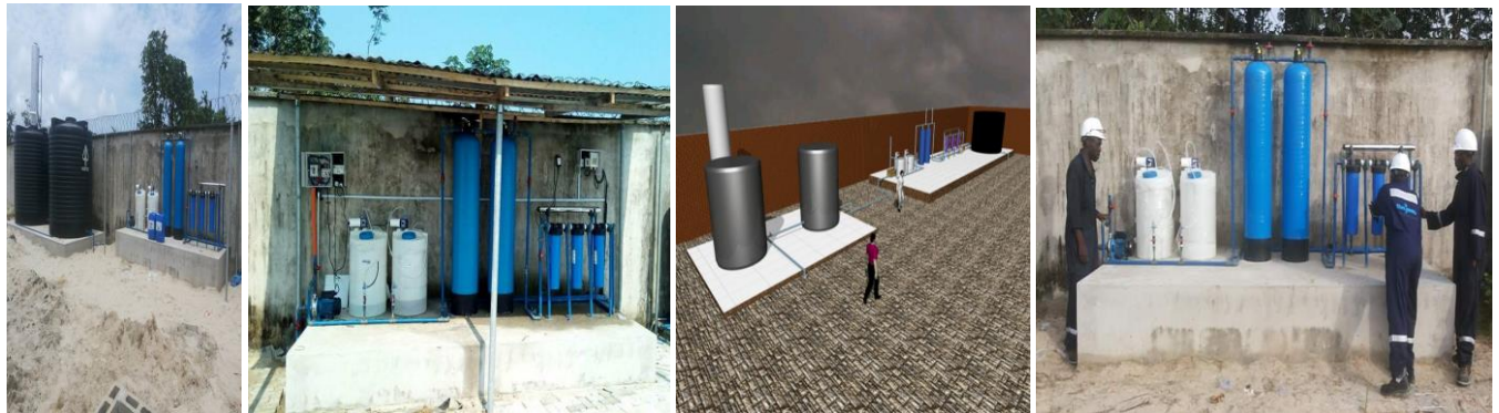
GREEN ENERGY INTERNATIONAL LIMITED/LEKOIL WATER TREATMENT PLANT (WTP) DESIGNED AND INSTALLED AT OTAKIKPO OILFIELD, ANDONI RIVERS STATE, NIGERIA BY MACJAMES.
