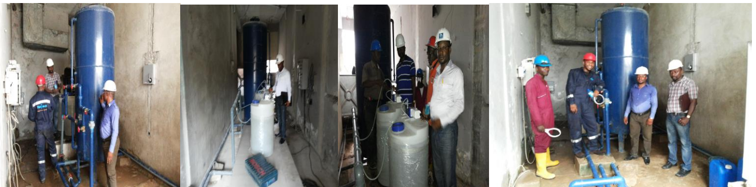
PHOTOS OF CENTRAL BANK OF NIGERIA; CALABAR BRANCH WATER FACILITY REDESIGN, REHABILITATION AND MAINTENANCE BY MACJAMES IN PARTNERSHIP WITH REAL-REPHIL SOLUTIONS LIMITED
