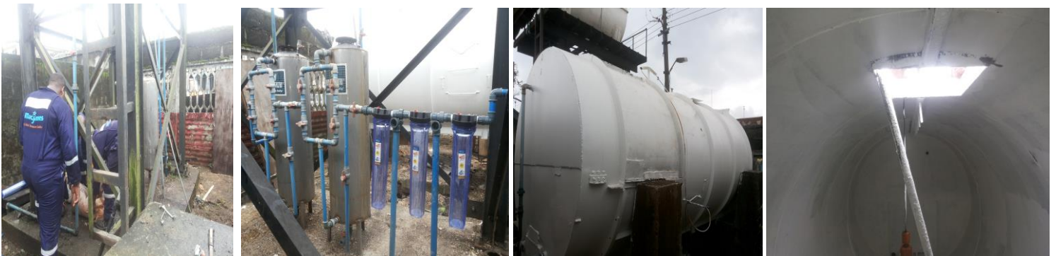
SeWa WEST AFRICA LIMITED FACTORY AND OPERATIONAL BASE DRINKING WATER TREATMENT PLANT REHABILITATION, RAW WATER HOLDING TANK ANTI-CORROSION TREATMENT, WATER QUALITY CHECK, AND DRINKING WATER TREATMENT, IN BOROKIRI, PORT HARCOURT, NIGERIA, CARRIED OUT BY MACJAMES WATER TECHNOLOGY.
