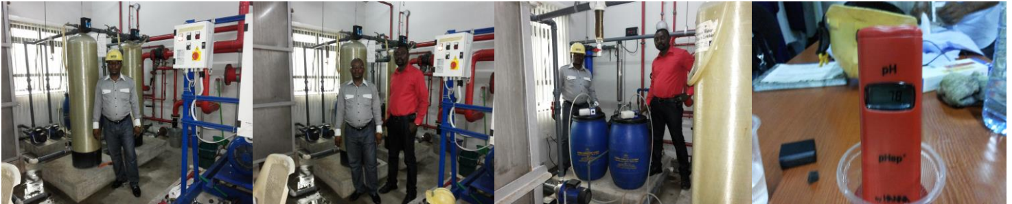
DURING CENTRAL BANK OF NIGERIA, UYO BRANCH WATER FACILITY MAINTENANCE AND WATER TREATMENT, CARRIED OUT BY MACJAMES IN PARTNERSHIP WITH REAL-REPHIL SOLUTIONS LIMITED.
