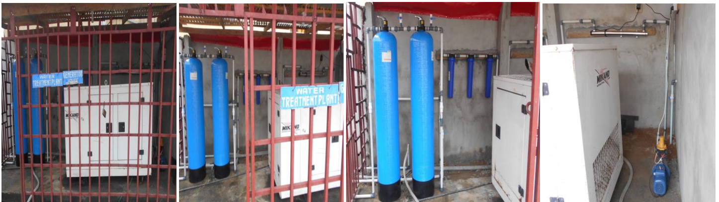
MACJAMES FACTORY WATER TREATMENT PLANT DESIGNED AND INSTALLED BY MACJAMES TO DE-IONIZE, DISINFECT, PURIFY, ADJUST PH AND PERFORM MULTIMEDIA AND MICRON FILTRATIONS
